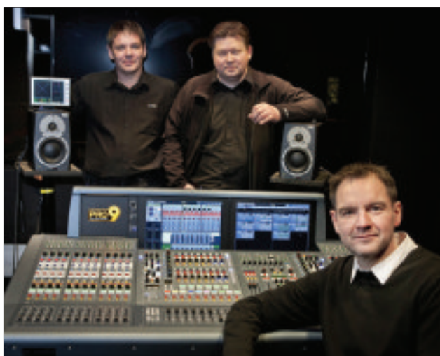
L-R: Gunnar Gunnarsson, Kristján Magnússon (project managers for Exton) and Ingvar Jónsson (Harpa technical manager of sound engineering) with one of the four Midas PRO9 consoles.
